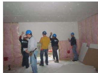
The Cementation Canada team and homeowner Kirsten Simpson hang drywall in the living room
